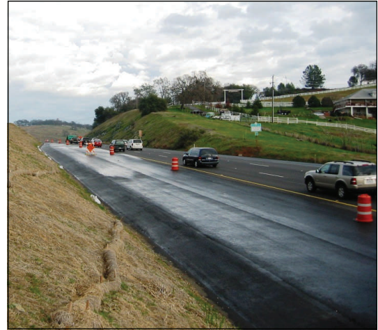
US 50 HOV Lane Phase 1 in Progress (El Dorado County Line to Bass Lake Road)
