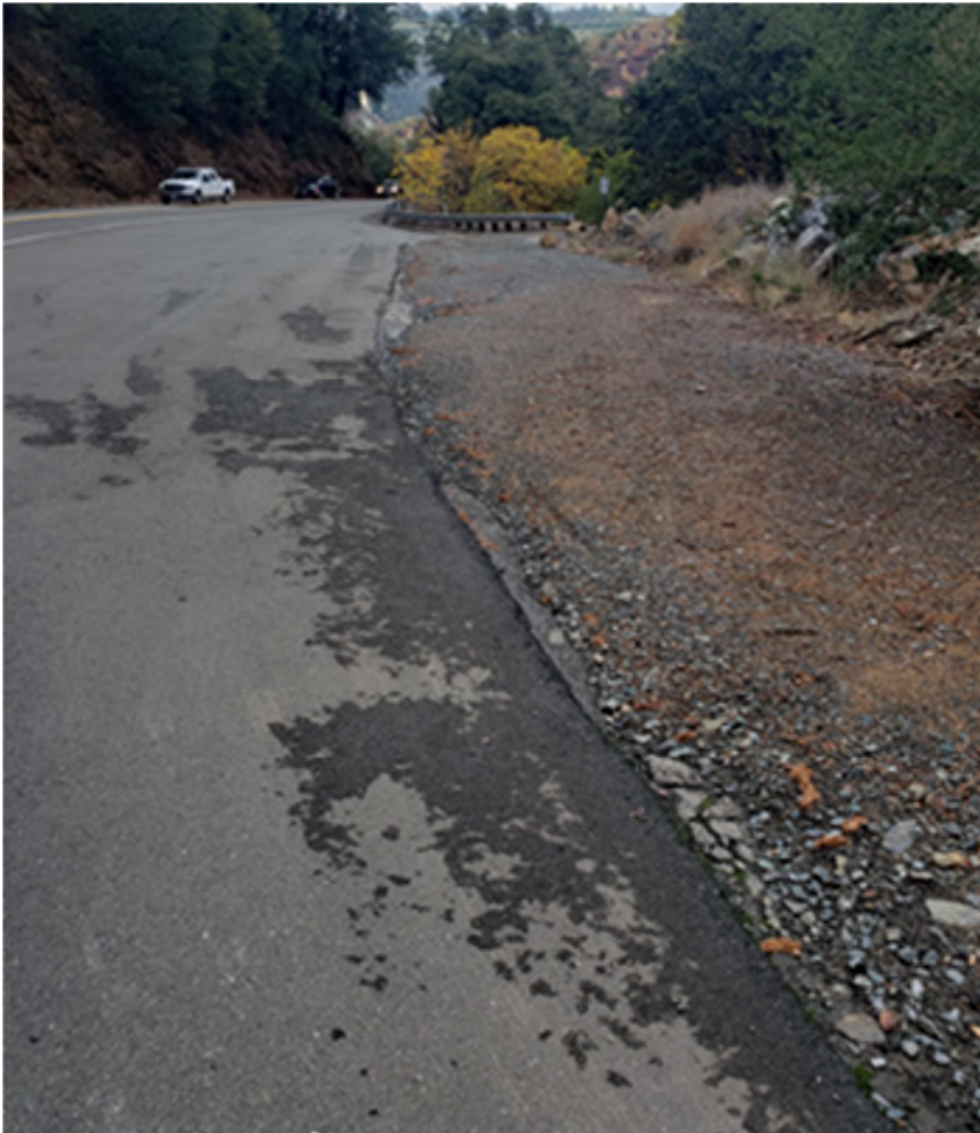
FIGURE 52: PHOTO OF SR 49 PARKING NEAR PM 35.5 EASTBOUND
