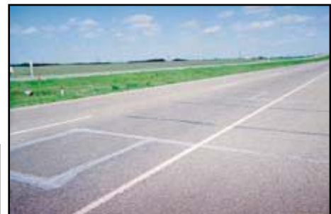
Figure 7 Loop Sensor in Roadway
