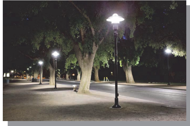
Contemporary LED street lights with directional shielding and placed to accommodate street tree canopies.
