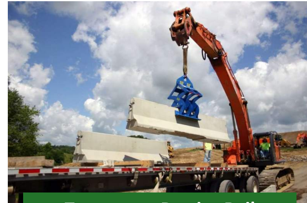
Temporary Barrier Rail
